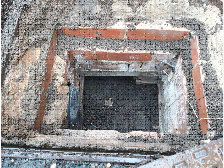
Highway drainage severely undermaintained reducing flow
