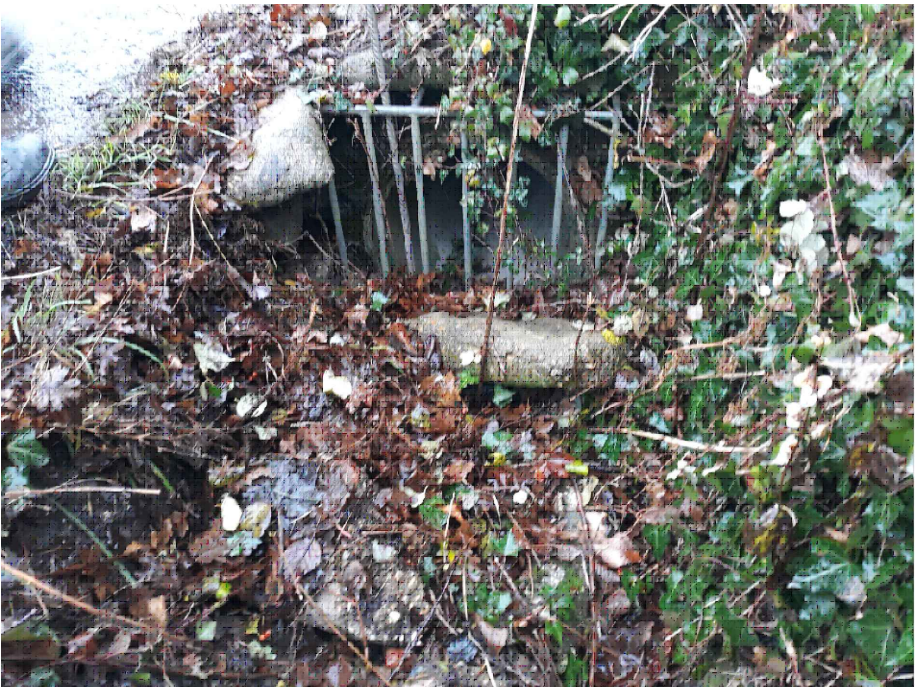
Concrete sandbag headwall collapsing and reducing flow into sewer
