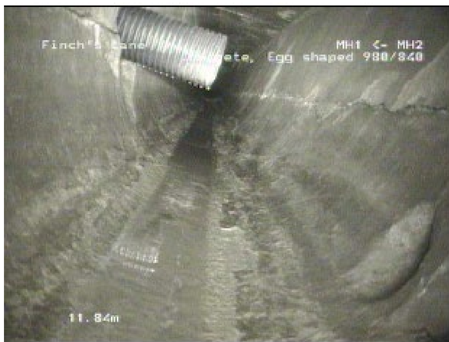
Figure 3.2 – Protruding connections into the sewer
