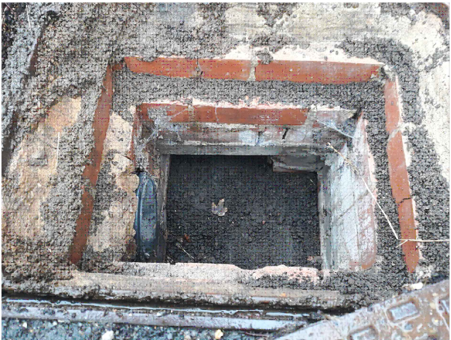
Highway drainage severely undermaintained reducing flow
