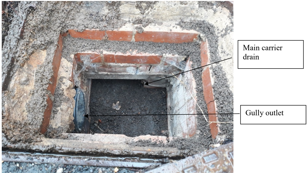
Figure 3.5 – Partially Blocked Highway Drainage
