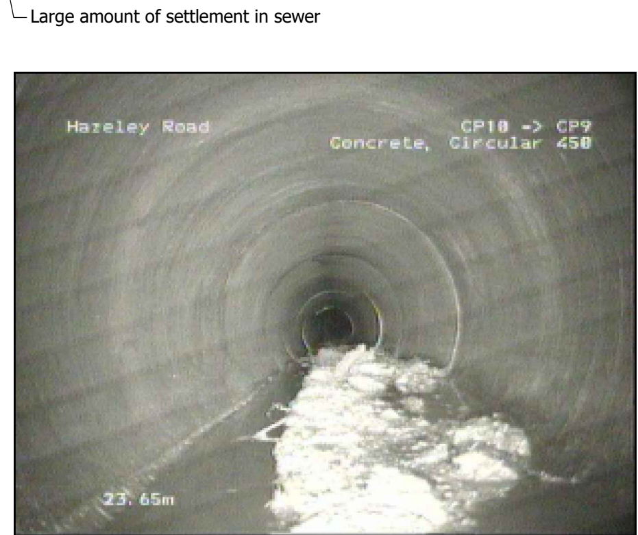
Large amount of settlement in sewer
