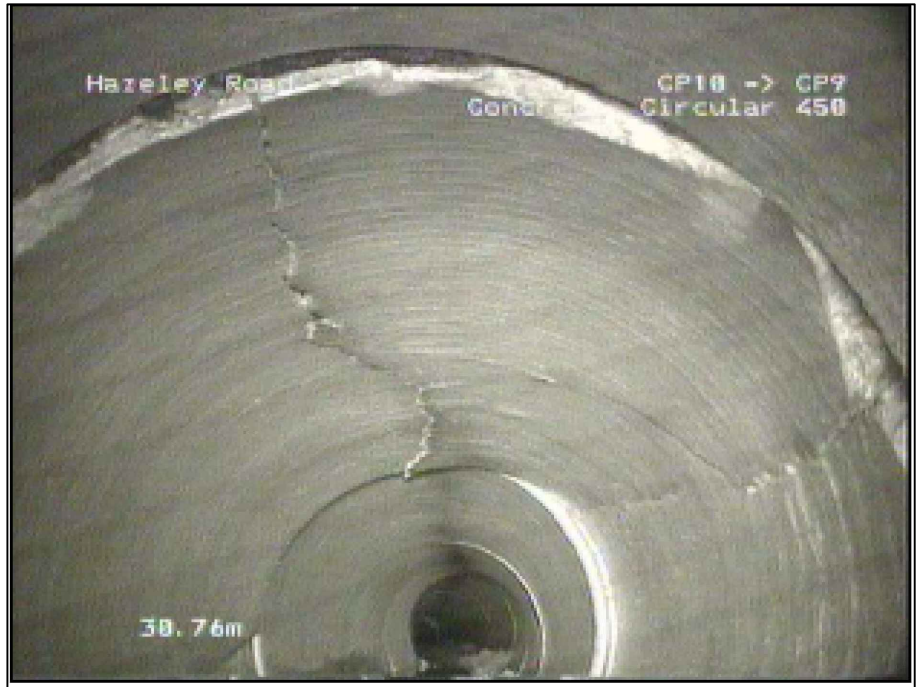
Longitudinal cracking in top of sewer
